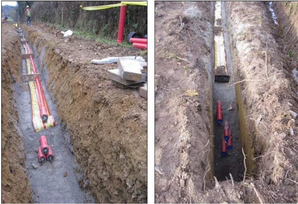
Plate 4-8 Typical Cable Trench View
